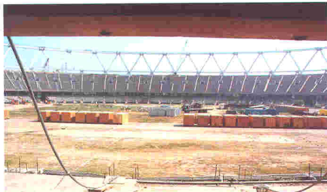
Still a lot of work to do inside the Jawaharlal Nehru Stadium where the Commonwealth Games ceremonies and track and field events will be held
