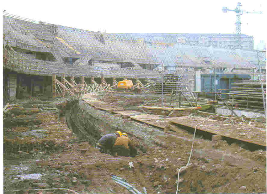
Under grey falling skies and a bitterly cold Alpine wind, Italian workmen put a new face on the Stadio Olimpico, the venue for the Games’ opening and closing ceremonies
