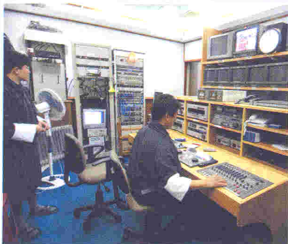
BBS control room
